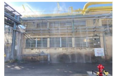
Operational water curtain
