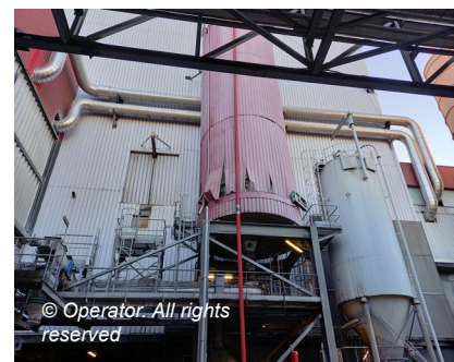
Damaged RPIFW silo
